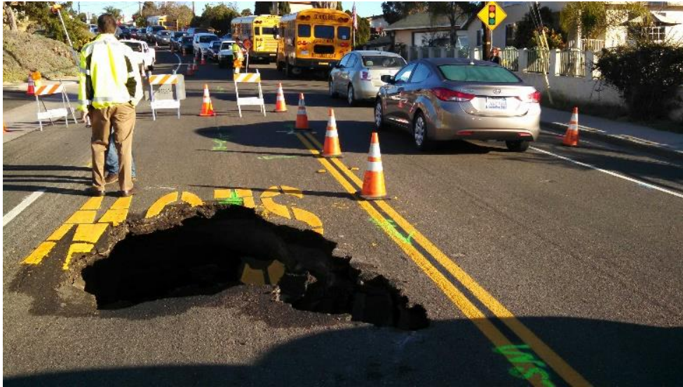
Figure 4-2 Sinkhole Caused by Pipe Failure on Oleander Ave near Valle Lindo Elementary School
