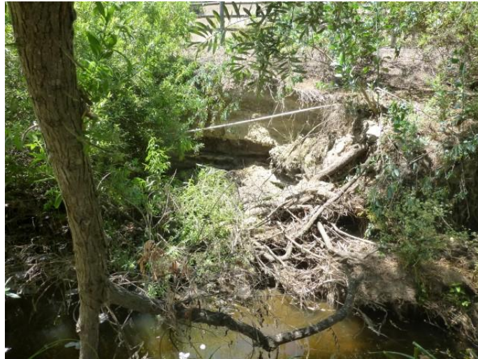
Figure 2-6 Natural Channel along Telegraph Canyon with Erosion Problem
