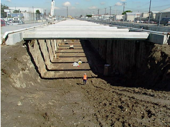
Stage 1: Excavation of the trench after installation of piles and top struts
