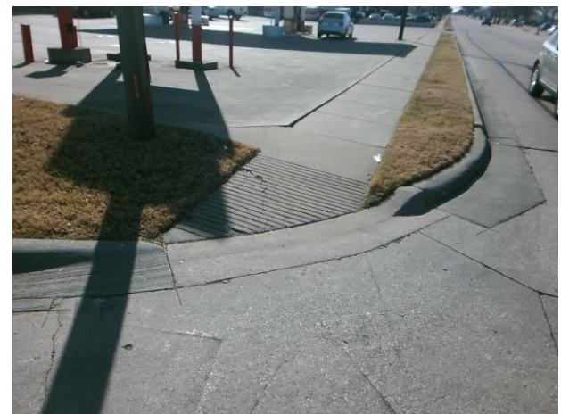
Curb Ramp Cross Slope
