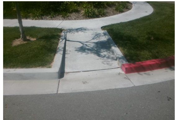
Curb Ramp Detectable Warning Surface-Missing
