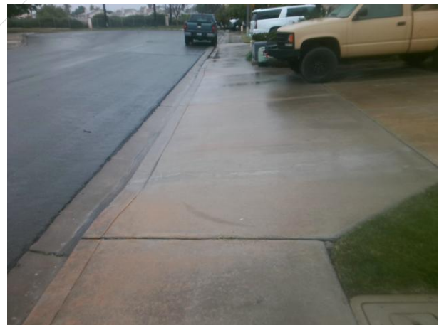
Steep Cross Slope - Driveway
