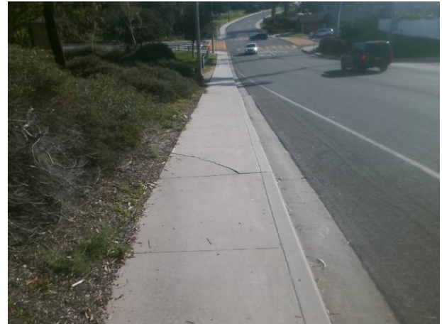
Sidewalk Changes in Level (Heaves)
