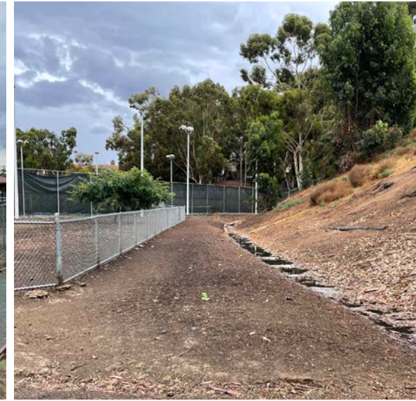
Drainage along slopes
