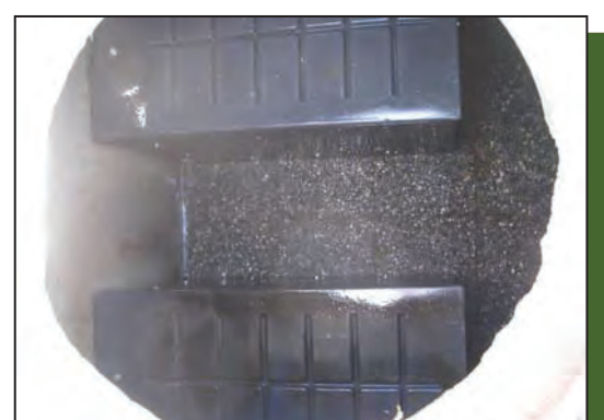
Fully cleaned separation chamber.
