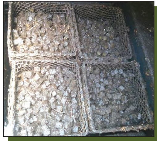
Inside cartridges showing media filters ready for replacement.
