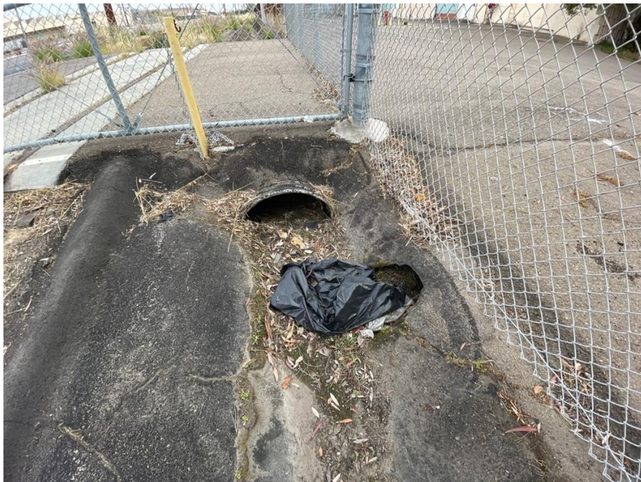
Photo 4. View of culvert and asphalt drainage that occurs west of project Planning Area A and east of Planning Area B-1 and Planning Area B-2.
