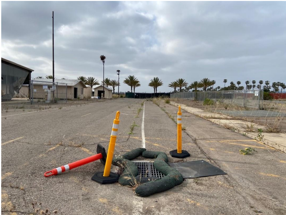
Photo 10. View facing southeast on the western side of the project site showing a stormwater collection grate.
