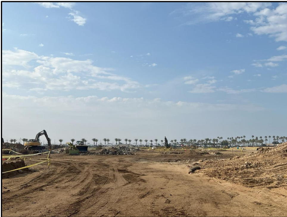
Plate 14: Overview of the project, showing heavy equipment and construction activity, facing south.
