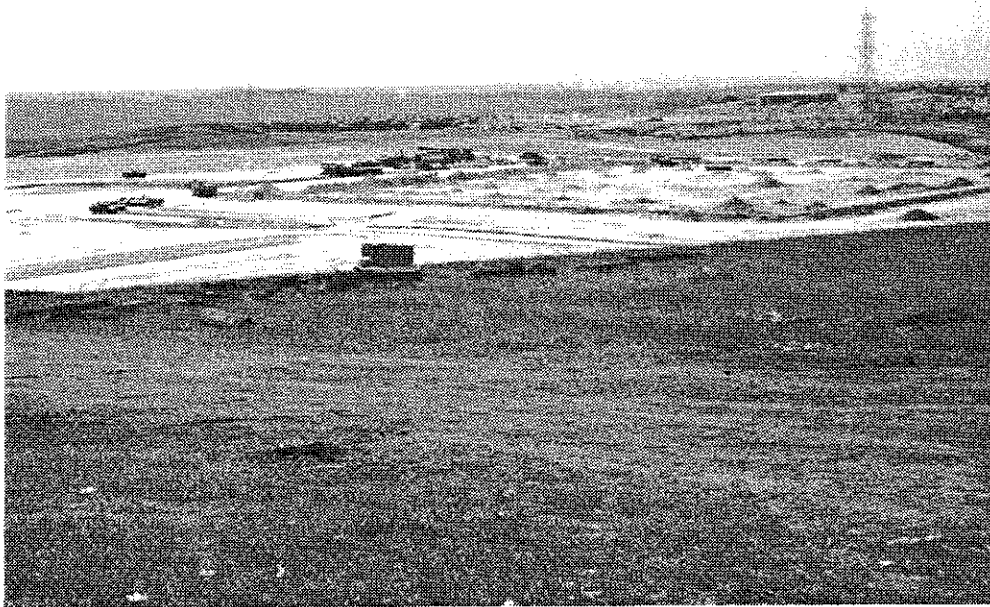
PHOTO F - Construction Underway at Eastgate Technology Park on Southern Boundary of Salt Creek Ranch. Eastlake Greens Development is in Background. On Clear Days the Ocean can be Seen from this Location.
